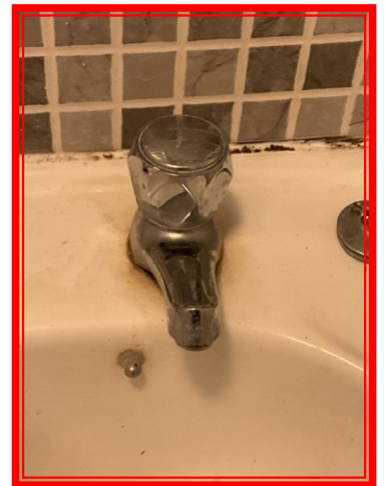
4.10.1 Stains and mould visible .
