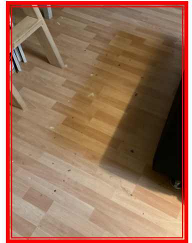
5.10.1 Paint marks and scuffs to floor throughout .
