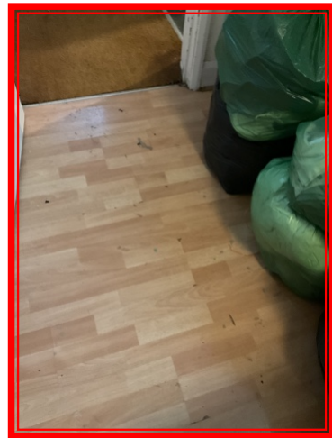
5.10.1 Paint marks and scuffs to floor throughout .
