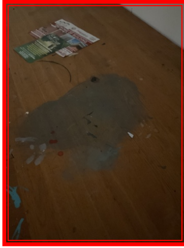
5.15.1 Multiple paint marks visible .
