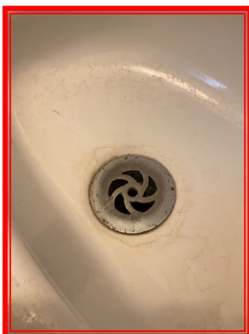
2.10.1 Minor staining present .
