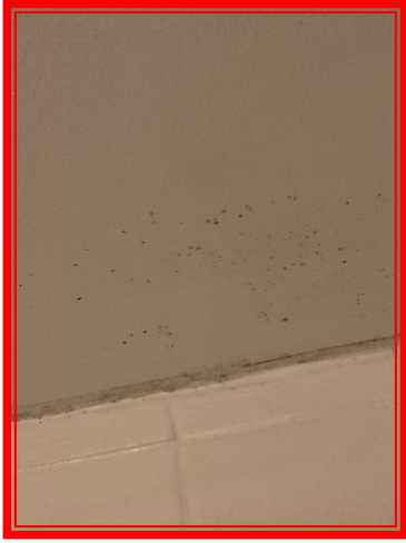
4.2.1 Minor mould above bath .
