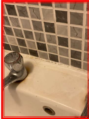
4.11.1 BATHROOM/ BATH/ BATH Stained throughout .
