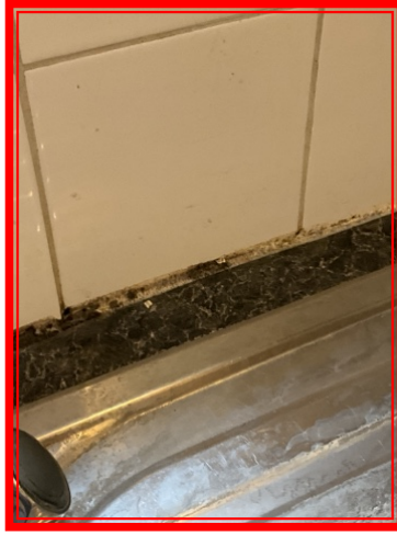
3.13.1 Mould to mastic around edges .
