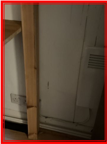
5.4.1 Damage to walls throughout, large hole to RHS of windows .
