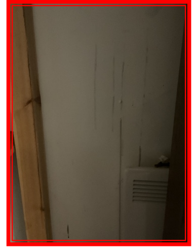
5.4.1 Damage to walls throughout, large hole to RHS of windows .
