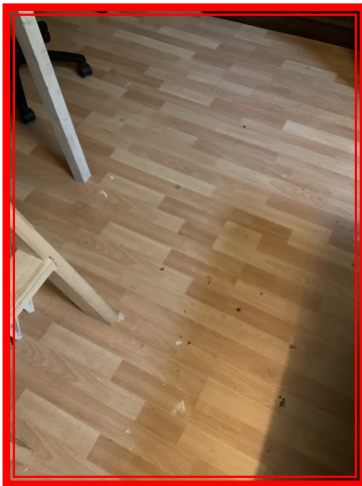
5.10.1 Paint marks and scuffs to floor throughout .
