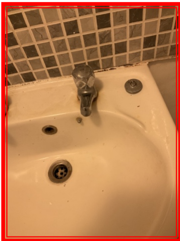
4.10.1 Chain from plug missing .
