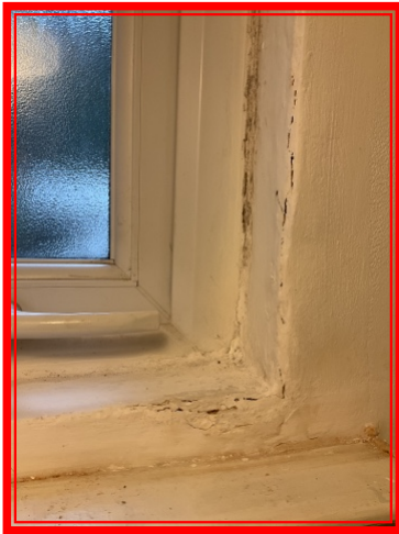
4.6.1 Signs of wear to edges .
