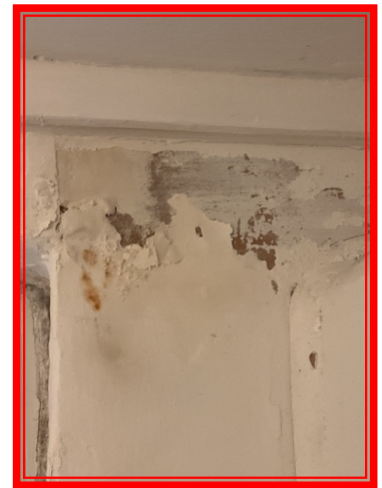
4.5.1 Marks and signs of wear to painted and tiled sections .
