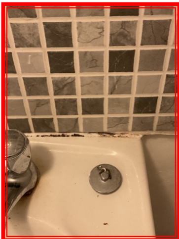
4.10.1 Stains and mould visible .
