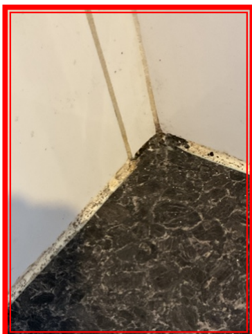
3.13.1 Mould to mastic around edges .
