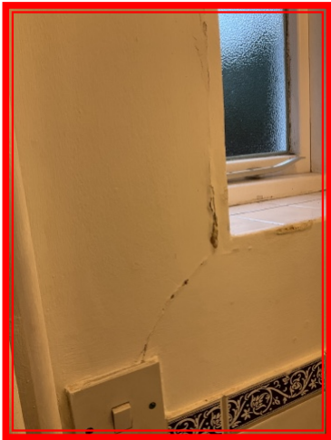
2.4.1 Cracks to LHS of window .
