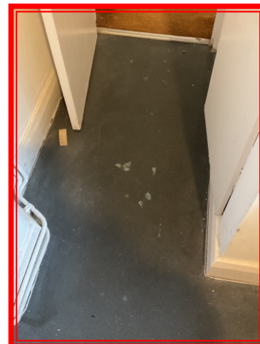
3.11.1 White stains visible .
