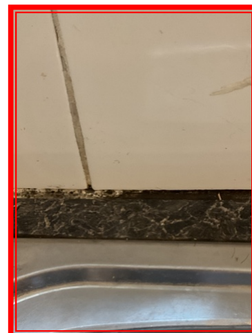
3.13.1 Mould to mastic around edges .
