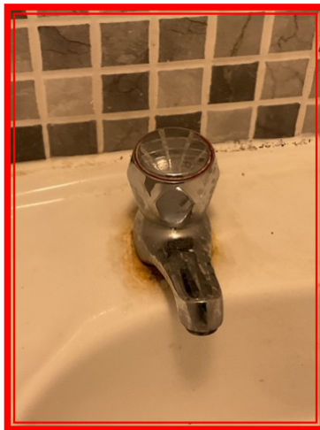
4.10.1 Stains and mould visible .
