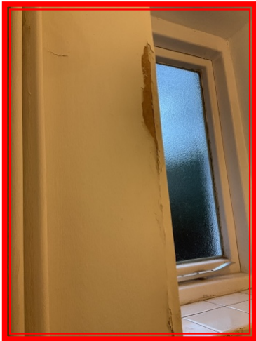
2.4.1 Cracks to LHS of window .
