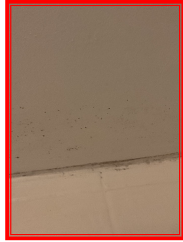
4.2.1 Minor mould above bath .
