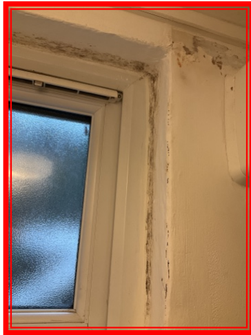
4.6.1 Signs of wear to edges .
