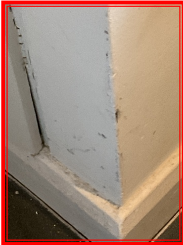
3.5.1 Marks and signs of wear to lower sections visible .
