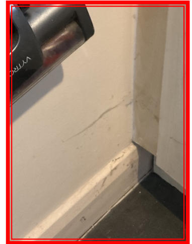
3.5.1 Marks and signs of wear to lower sections visible .
