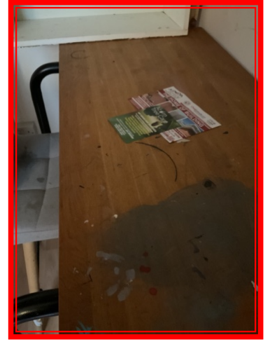
5.15.1 Multiple paint marks visible .
