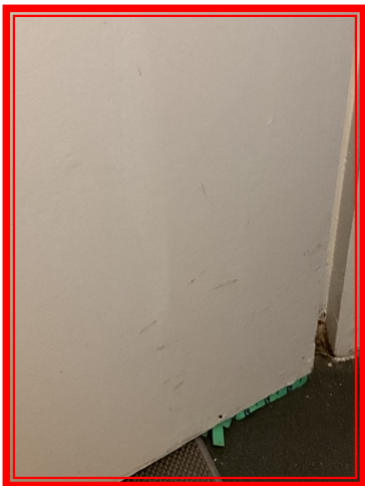
4.1.1 Minor marks and cracks visible to lower sections.
