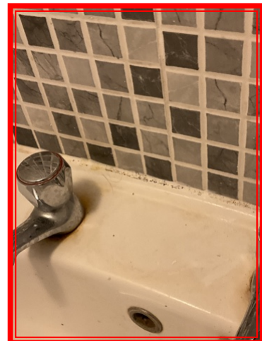
4.10.1 Stains and mould visible .
