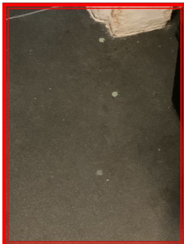
3.11.1 White stains visible .
