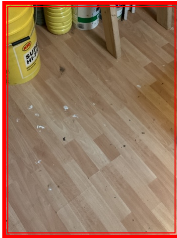
5.10.1 Paint marks and scuffs to floor throughout .
