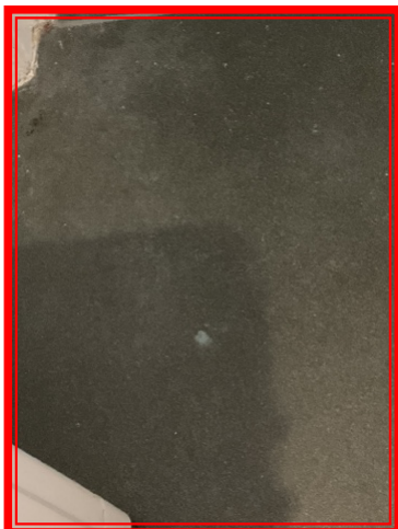
3.11.1 White stains visible .
