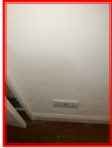
1.4.1 Marks and signs of wear to lower sections .
