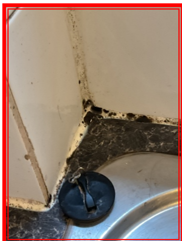
3.13.1 Mould to mastic around edges .
