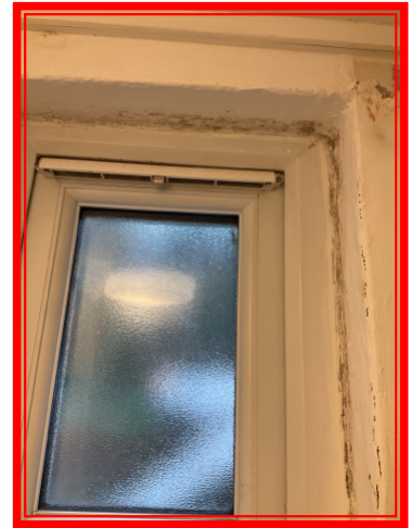
4.6.1 Signs of wear to edges .
