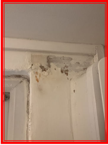
4.5.1 Marks and signs of wear to painted and tiled sections .
